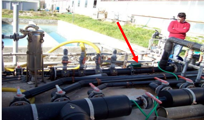
Figure 2: An Agriflow unit installed on the incoming water to the whole plant.
