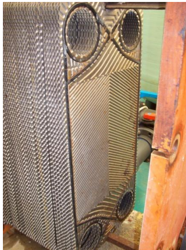
Figure 6: A heat exchanger protected against limescale by Agriflow. Instead of twice-yearly acid washes, the exchanger is hosed down once a year as part of routine maintenance.
