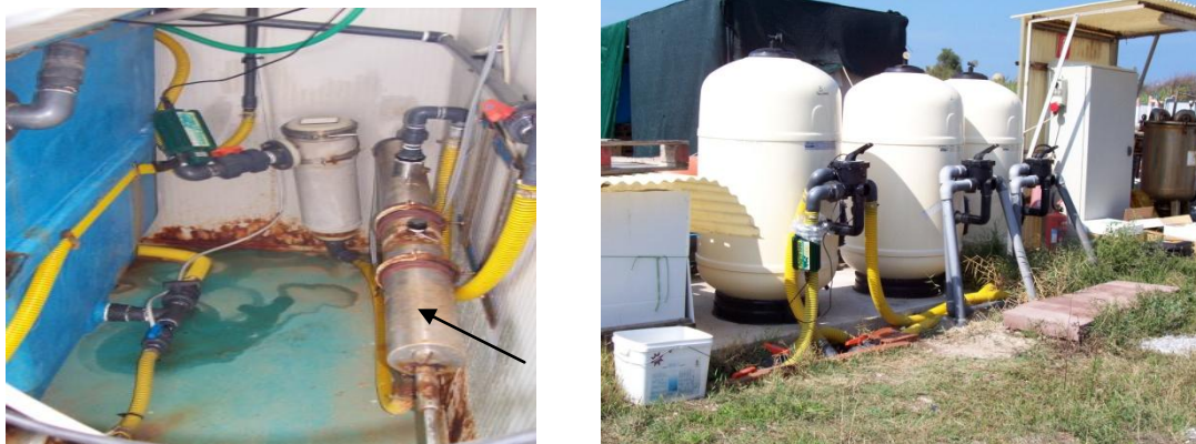
Figure 9: External water storage tanks also had their UV protection replaced with Agriflow.
